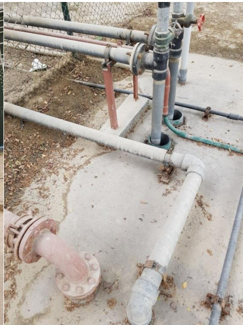
Fig 2.3 (Pipe from water tank)
