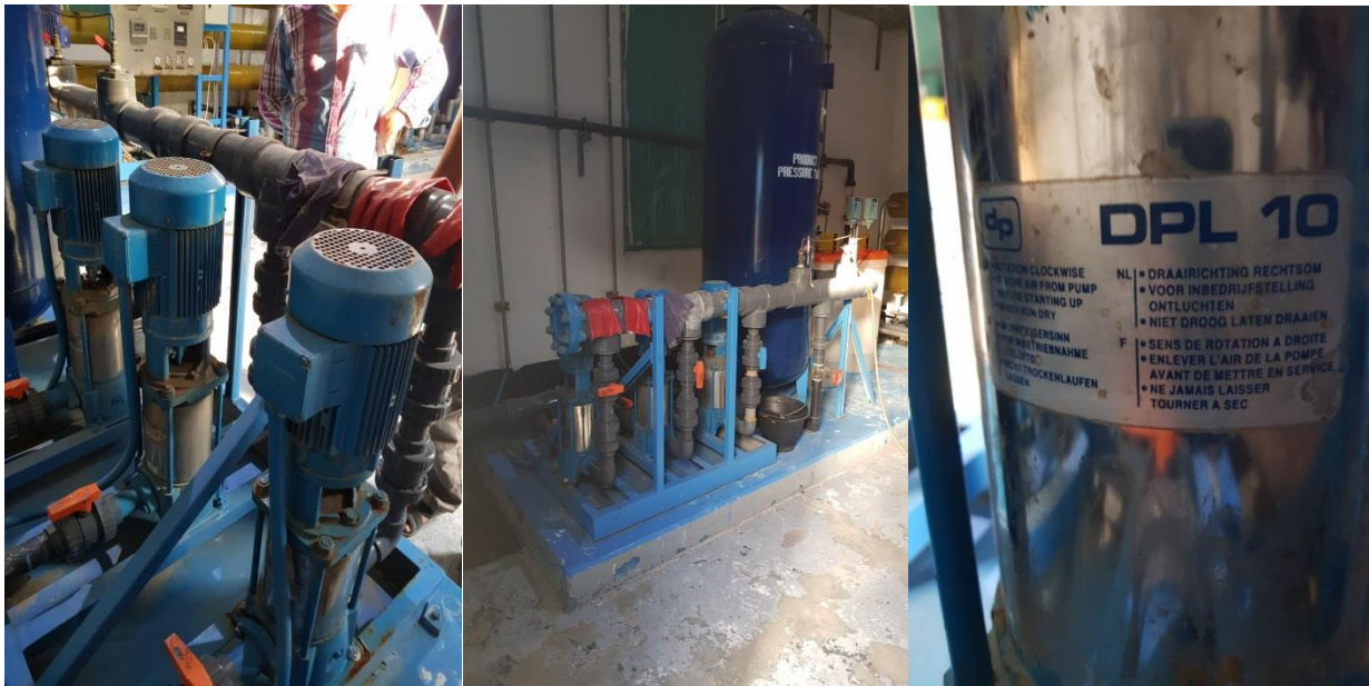
Fig 2.4 (Pumps side view) Fig 2.5 (Pumps Back View) (Fig 2.6 (Pumps Powering the System))
